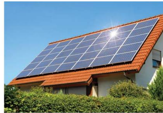
▲ Figure 12 A domestic photovoltaic panel system.
